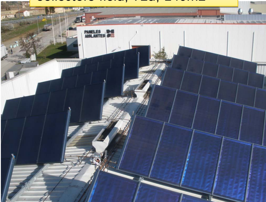
Collectors field, 72u, 140m 2
