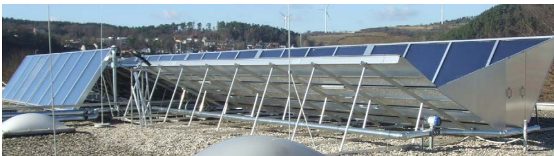
Picture 1: Collector field on the roof of the laundry. Reference flat-plate collectors (glass-foil, front) and newly developed RefleC-collectors (back), Source: S. Heß, Fraunhofer ISE
