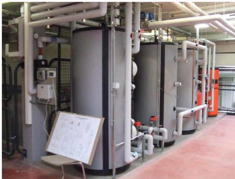
Picture. 2: Buffer storages of the solar thermal system with control unit and piping. In the front is the primary storage, in the middle the two secondary storages and in the background (orange) the buffer storage to supply the washing machines with process water.
