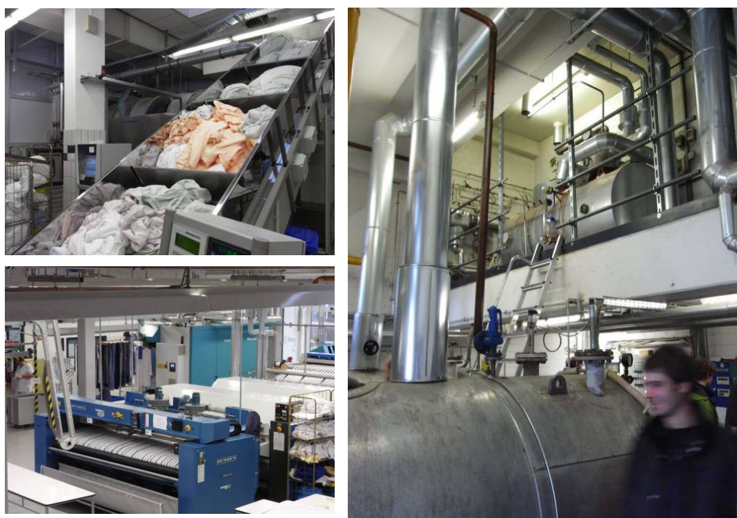
Picture. 3: Washing plant of the laundry, (left side top), ironing machine (left side bottom) and steam boiler room (right) with steam boiler (front) and feed water tank (upper floor).
