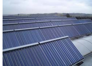
Source: Sotec Solar, Germany
