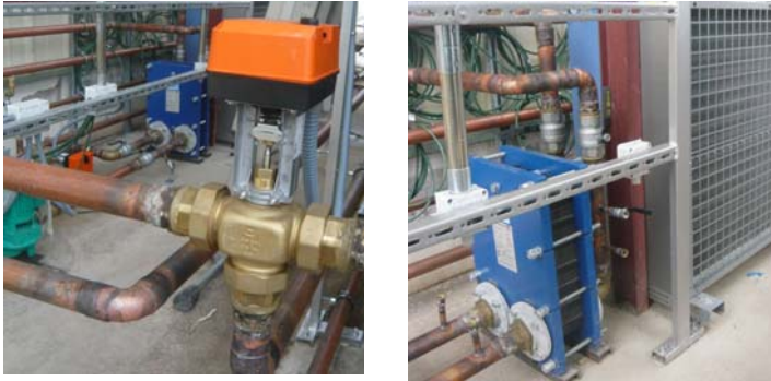
3 ways-valve and exchanger
