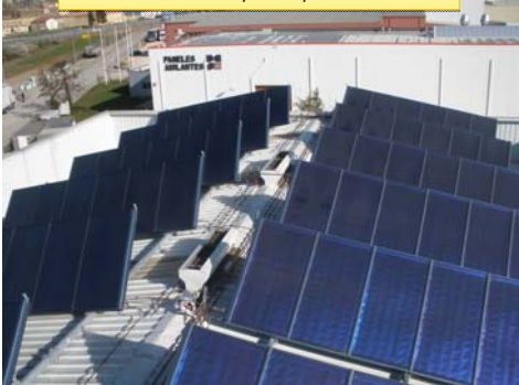
Collectors field, 72u, 140m2
