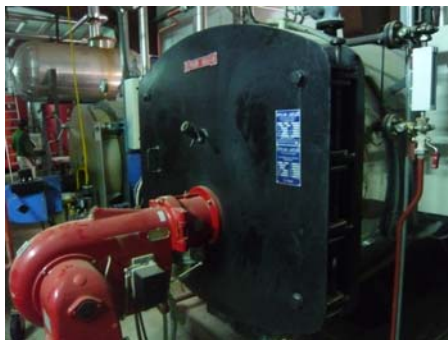
The old oil boiler, 1080 kW, 14 years
